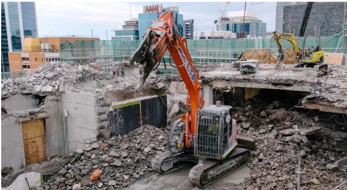
Figure 7: Structural Demolition on the top floor at the Victoria Cross Station Site
