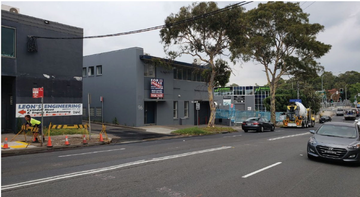
Figure 8-8 Viewpoint 2 – Current view (Note: The existing building on the site had already been demolished at the time of the preparation of this SDPP)
