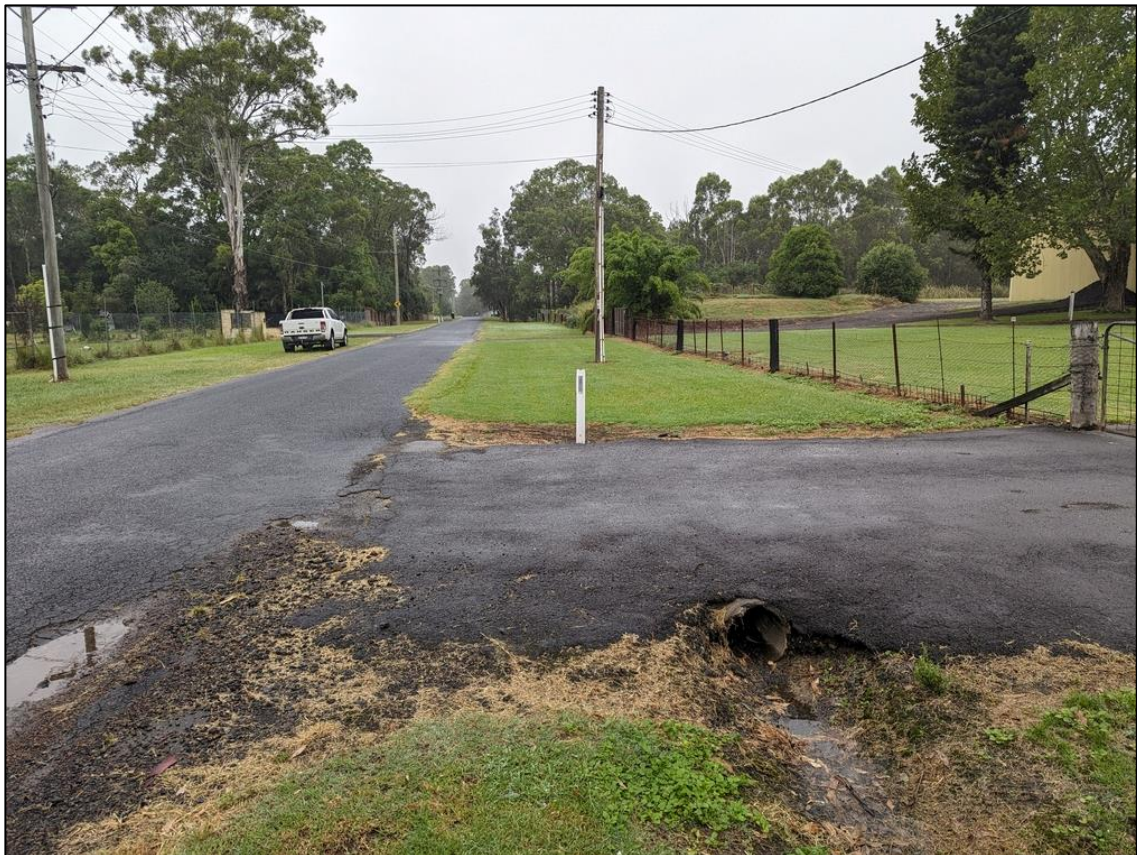
Photograph 8: Showing evidence of drainage pipes installed beneath driveways along Samuel Marsden Road.
