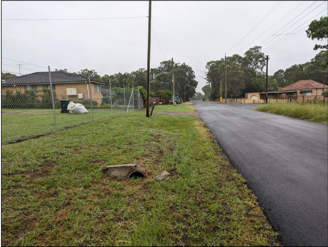
Photograph 11: Showing evidence of drainage channels within the road reserve.
